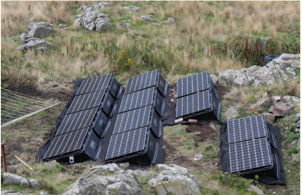
Plate 350. New solar panels. © Mark Oksien
