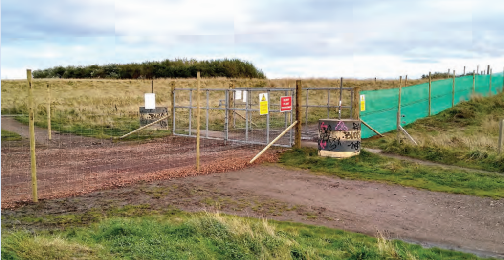
Plate 233. Work on creating the new wetland at Musselburgh means that pedestrian access will be restricted for over a year to allow heavy vehicles to pass, 2 November 2021. © Ian Andrews
