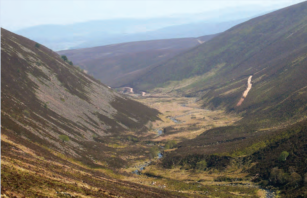
Plate 227. Hill track construction by a tracked excavator in May 2008 past the eyries on opposite side of the glen. © Alastair Pout
